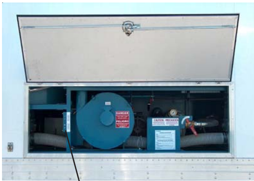
Vacuum & Blower 4 (2 per)
