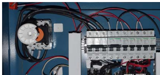
The fuse protection - breakers. (Illust. 16)
